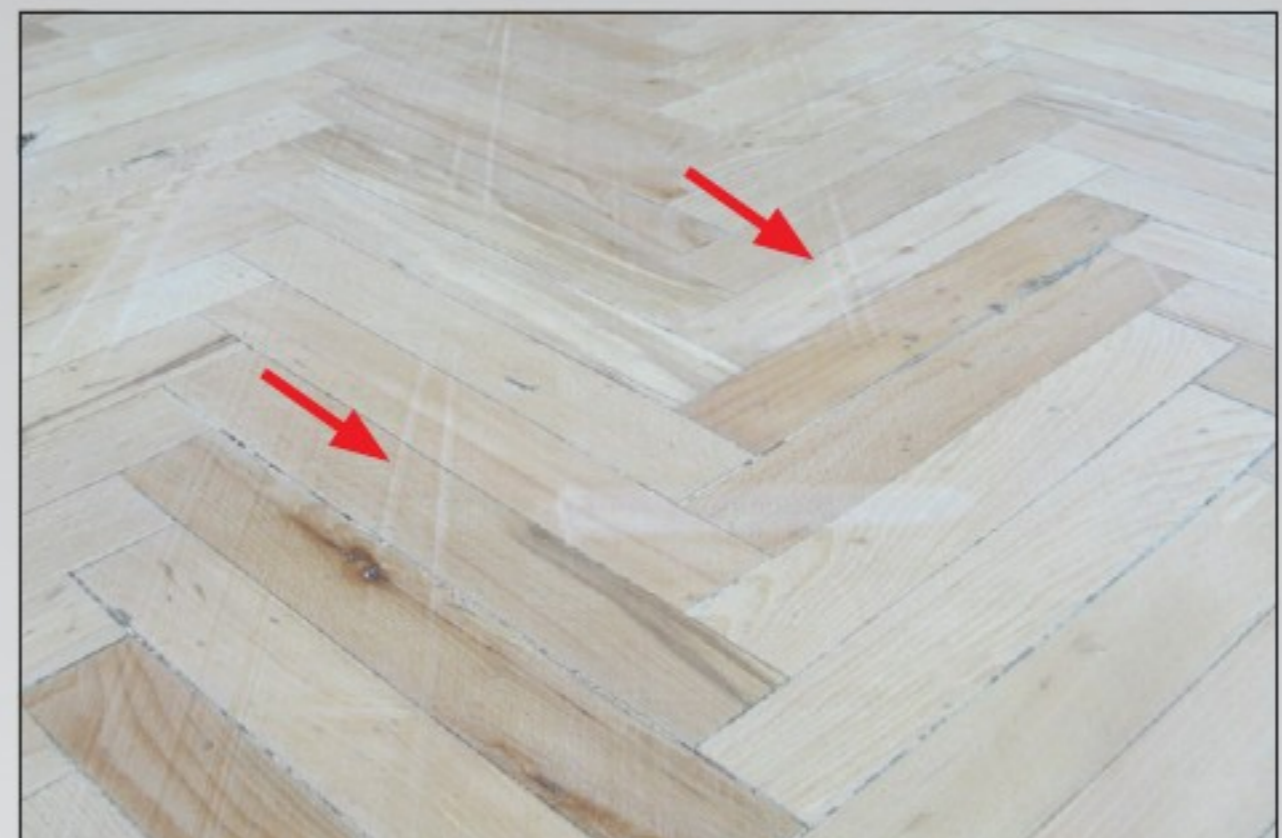
Pic. 4 Grooves in the floor
